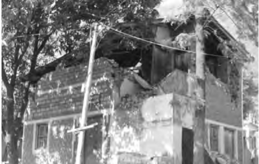
Figure 6.1 : A Damaged Building Due to an Earthquake
